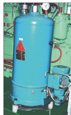
HDU 27/54 P for lube oil treatment
